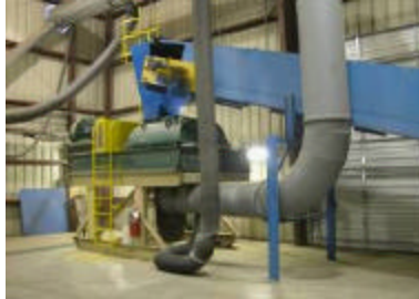
Enclosed infeed conveyor
