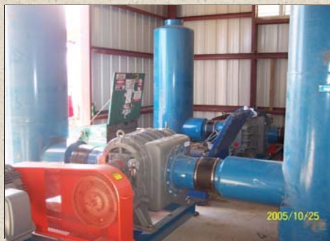
the blower room where it is sent pneumatically to ignite with coal.
